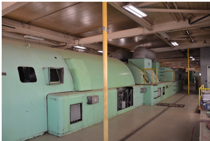
Figure 4 Unit 3 Allis-Chalmers Steam Turbine Generator
