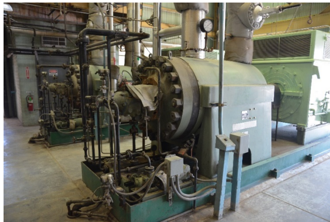
Figure 9 Unit 3 Allis-Chalmers Feed Pump
