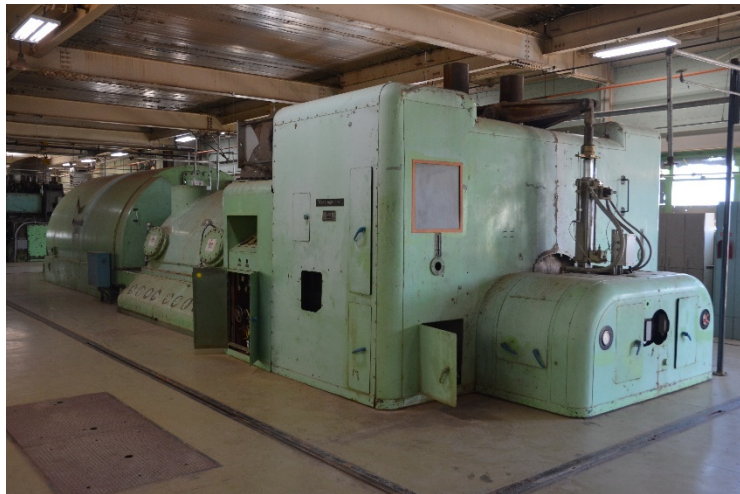
Figure 3 Unit 2 Westinghouse Steam Turbine Generator
